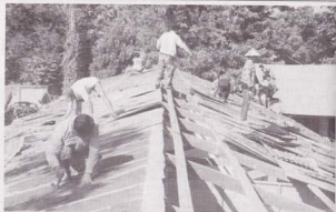
Villagers of Donekoi, in Sisattanak district replace the roof of the local primary school. The roof had not been replaced for 13 years and was in poor condition. The locals also cleaned the school grounds and did other maintenance.
